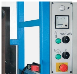
Low tension electrical panel
